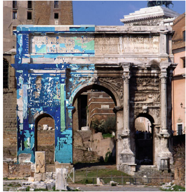
Conservation, Restoration, and Preservation in Classical Archaeology, Fig. 1 Arch of Septimius Severus in the Roman Forum, 1983. Table of stone's deterioration mechanisms. The documentation regarding the state of conservation of monuments has slowly become a fundamental instrument for the curator/restorer. (Pictures Nardi, Copyright CCA)
