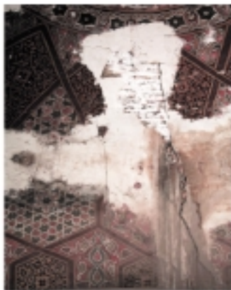
LACUNE, CRACKS, BREAKS
