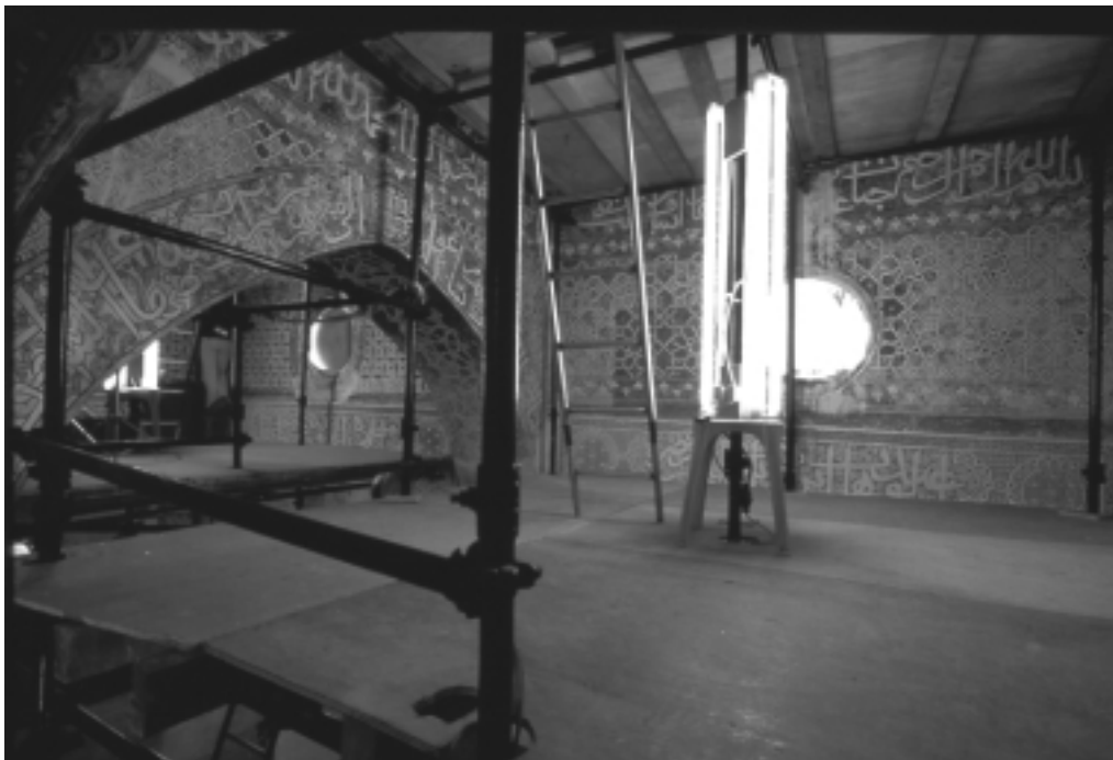
20 The scaffolding was equipped with an autonomous system for power and lighting.
