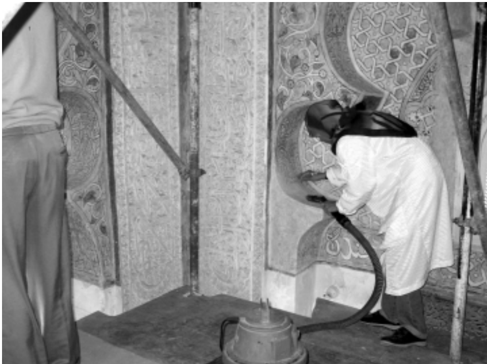
22. The future of the Amiriya is in the hands of a regular implementation of the maintenance program.
