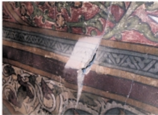
DETACHMENT OF INTONACO
