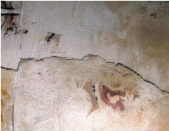
34. Dome 2. The intonachino (a second strata of intonaco ) covers traces incised with a compass to divide the surface of the first plastering into various decorative fields.
