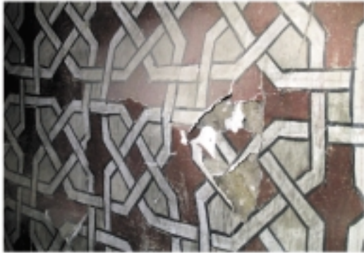
DETACHMENT OF INTONACO
