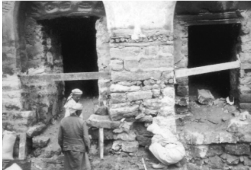
9. Rebuilding the lower sections of the arcades and piers was the first thing to be tackled.
