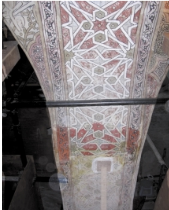
33. The underarch between domes 1 and 2 seems to show an area inaccessible when the original scaffolding covered it.
