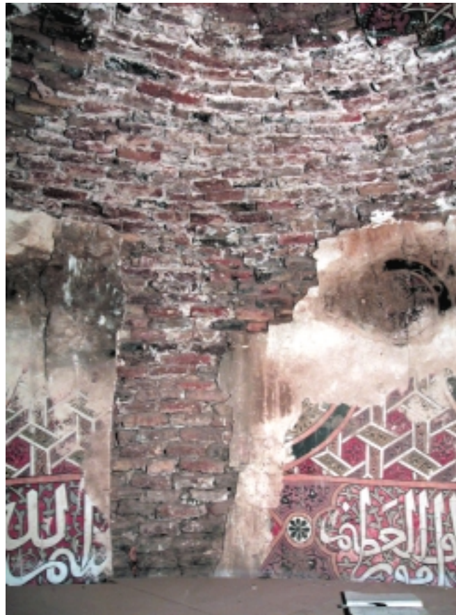
28. Dome 5. Detail of the brick structure in an area of missing plaster.
